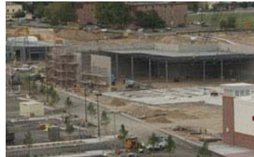
Construction at Havana Gardens is shown Aug. 25 near South Havana Street and East Mississippi Avenue in Aurora. Dick's Sporting Goods and Petsmart are planning to move into the development once it is complete. (Heather A. Longway/The Aurora Sentinel)
