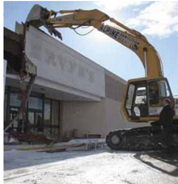
Mayor Ed Tauer watches the old Meryvn's marquee being torn down Jan. 8 during the demolition ceremony of the Buckingham Square Mall. (Photo by Heather A. Longway-Burke/The Aurora Sentinel)
