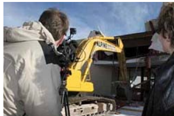
Charles Hack, videographer for Aurora 8, and Yasmine Marino, volunteer reporter with Aurora 8, cover the demolition ceremony of the Buckingham Square Mall on Jan. 8. (Photo by Heather A. Longway-Burke/The Aurora Sentinel)
