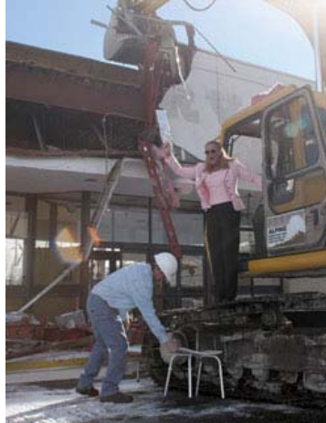
Heather A. Longway-Burke/The Aurora Sentinel City Council woman Molly Markert steps off the excavator, with help from Jim Gochis of Alpine Demolition, after helping demolish some of the Buckingham Square Mall Jan. 8 during the demolition ceremony of the Buckingham Square Mall.
