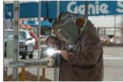
It takes a welder's mettle to meld the structural metal together for The Gardens on Havana. The Buckingham Square shopping center was razed, making way for the mixed-use project. (John Prieto, The Denver Post)
